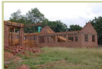
NEW CONSTRUCTION -- Following the principles of Shalom Zone training, Hilltop United Methodist Church in Sakubva, Zimbabwe, created its own construction company to build new facilities for Isheanesu, a program empowering women and men to become self-sufficient and their children to succeed academically. Construction costs for the new building to house classrooms, training programs and indigenous businesses are being underwritten by the Holston Annual Conference. A UMNS photo by Jane Malone. Photo number 02-76, Accompanies UMNS #113, 3/19/02
